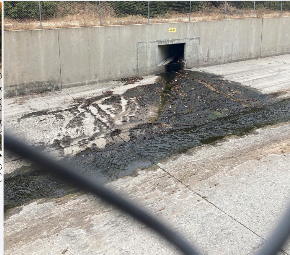
Dark muck flowing into the River
